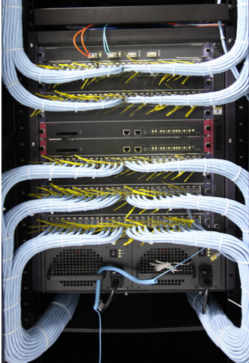
Figure 11-4 Network cable management
