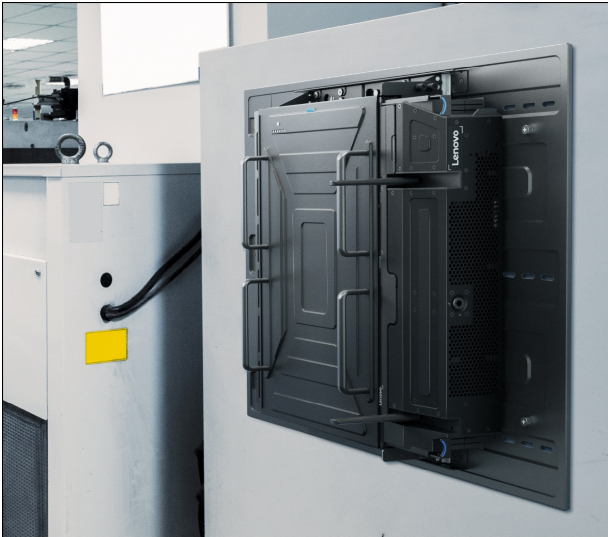
Figure 18. SE450 installed on a wall in a manufacturing environment
