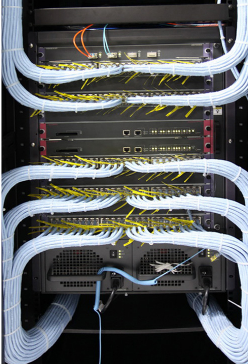
Figure 12-4 Network cable management
