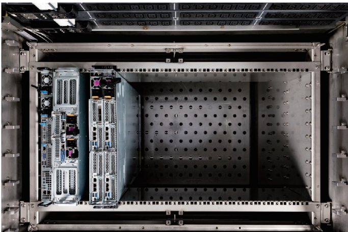
▲ Overhead view of A1P0-EB0 Tank
