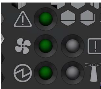
System Status LEDs* 5 Minutes After Power On
